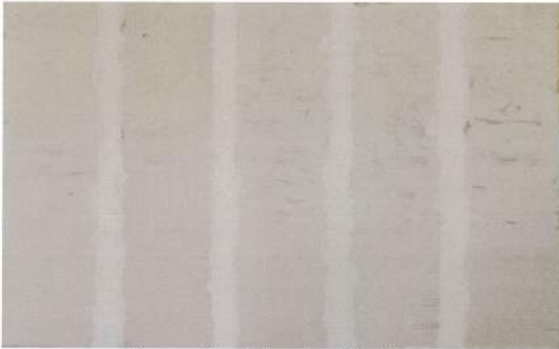
The exposed face of the specimen before the test
